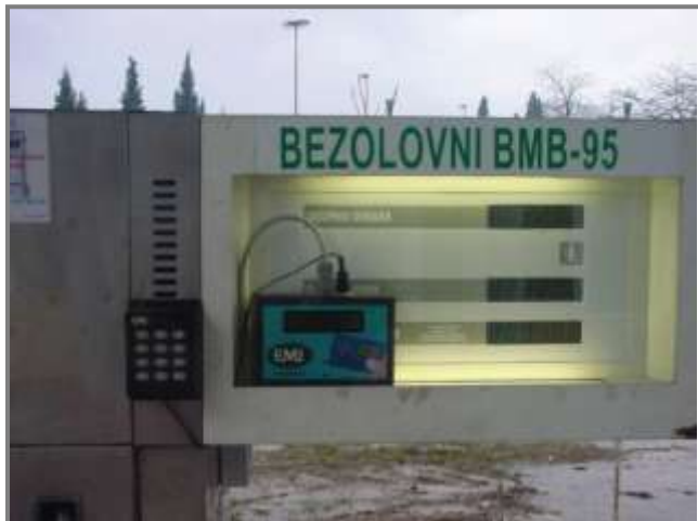
Figure 6: Dispense Controller and Keyboard Mounted on the Fuel Dispensing Device
